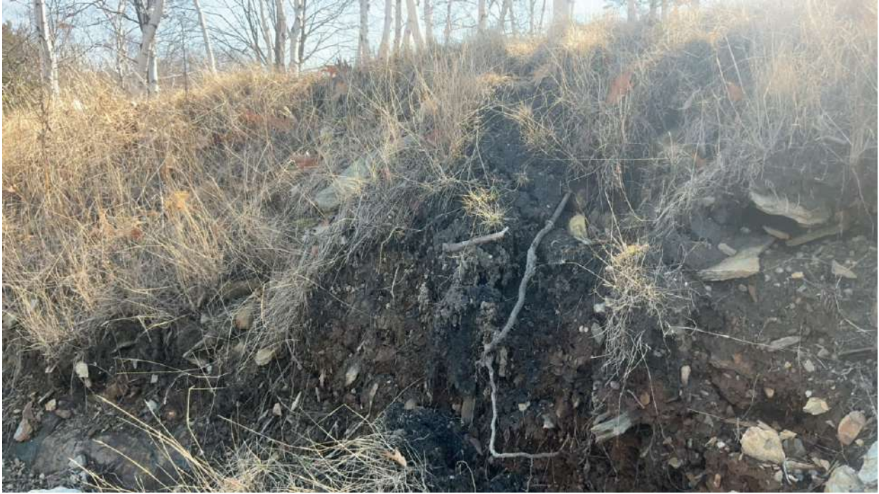
Figure 5: Soil erosion is visible above the top of the placed stone in this section of bank adjacent to the barge landing.
