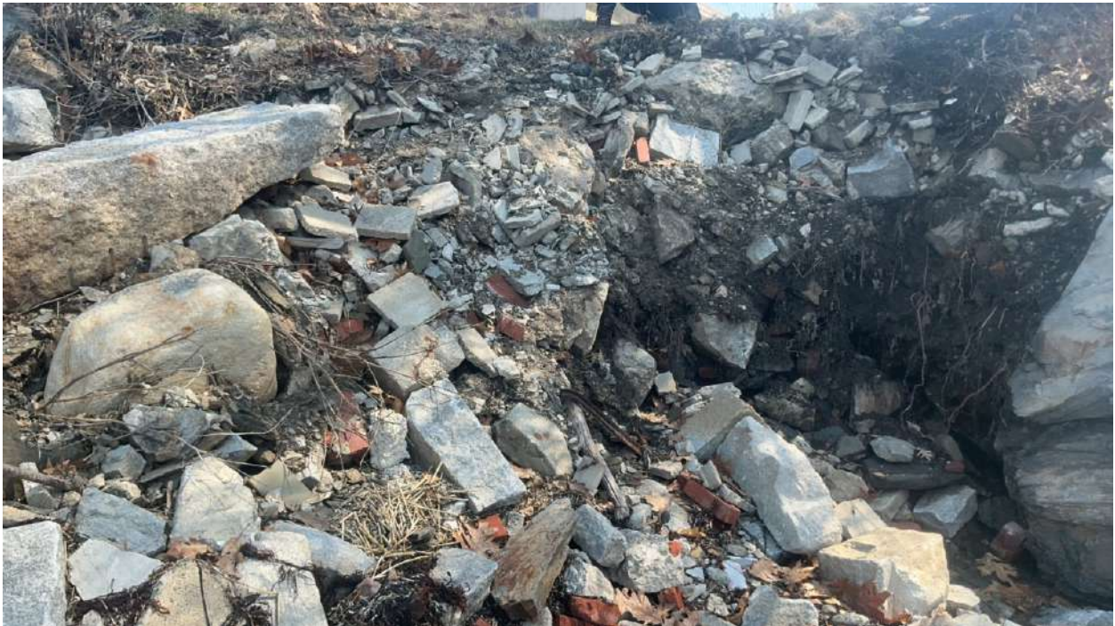
Figure 4: Water now drains from this section of bank after a drainage pipe failed. Bricks and debris are visible in the bank.
